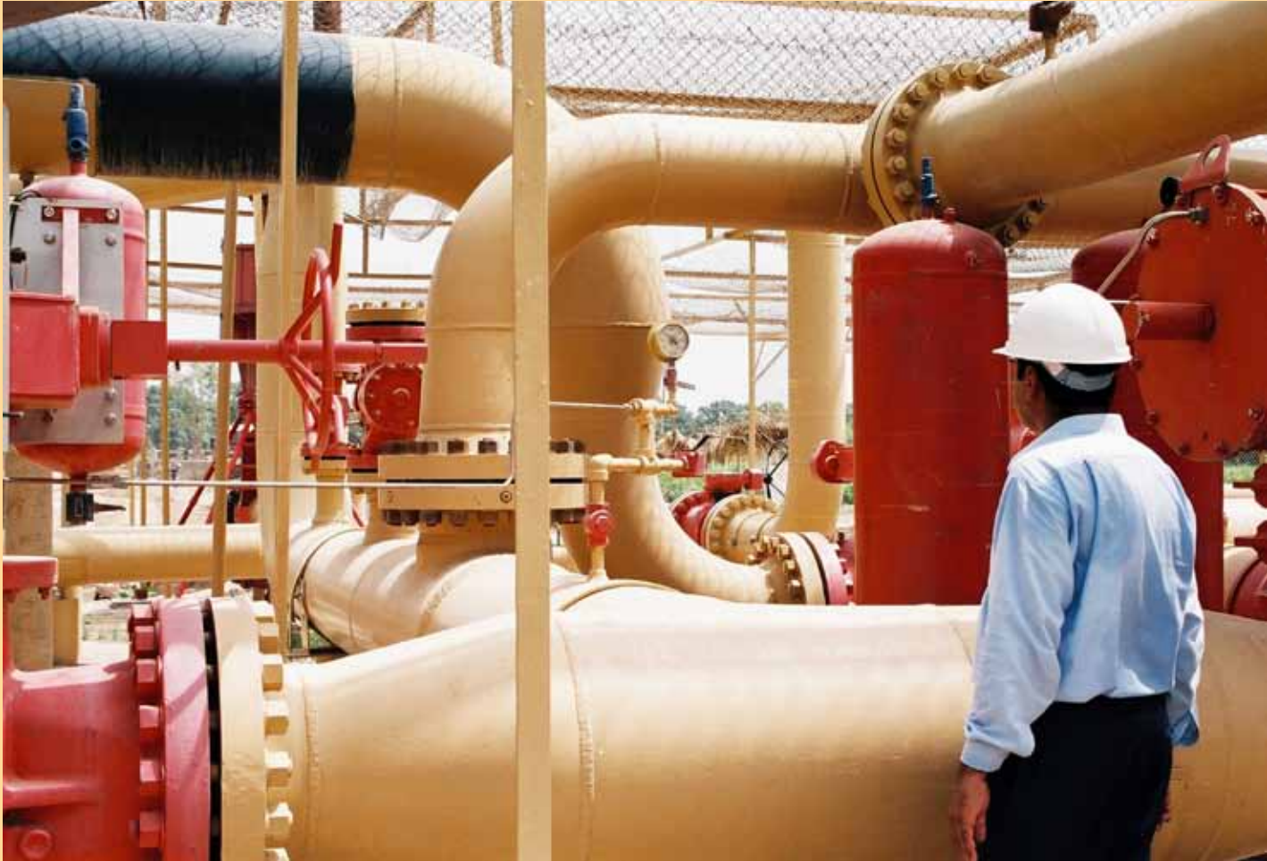
Valve Assembly – starting point 36” diameter Multan-Sahawal gas pipeline.
